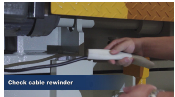
Check cable rewinder
