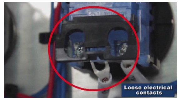
Checking electric point
