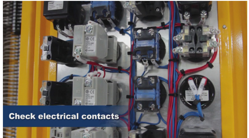
Checking electric poing
