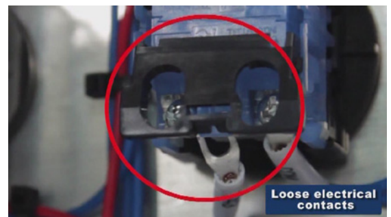
Loose electrical contacts
