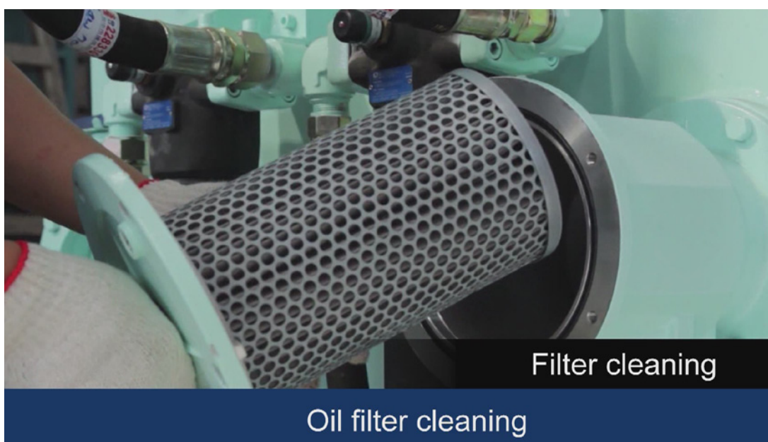
Oil filter cleaning
